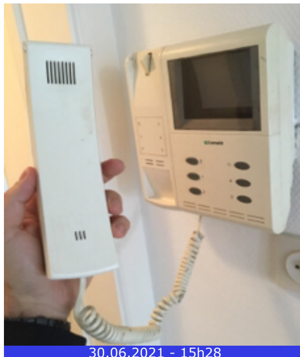
Photo 10 (Hall / Interphone / Etat d'usage)
