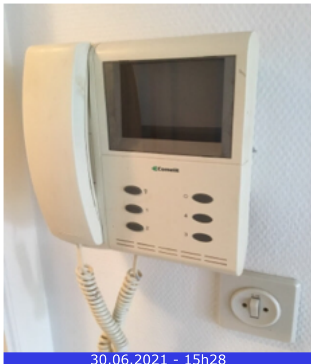
Photo 9 (Hall / Interphone / Etat d'usage)
